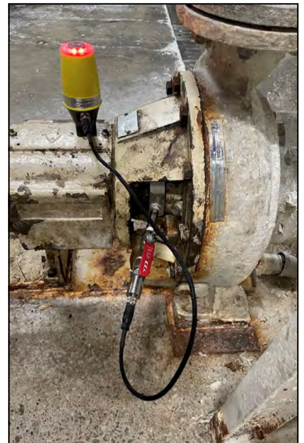
Chesterton Solution installed with Chesterton Connect Monitoring
