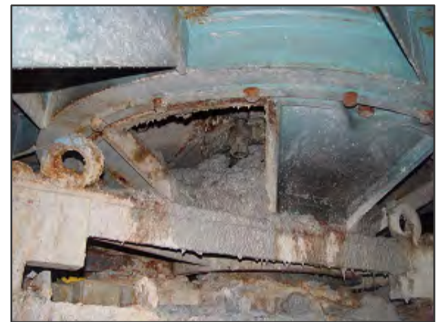
Before, damaged gearbox with leaked product
