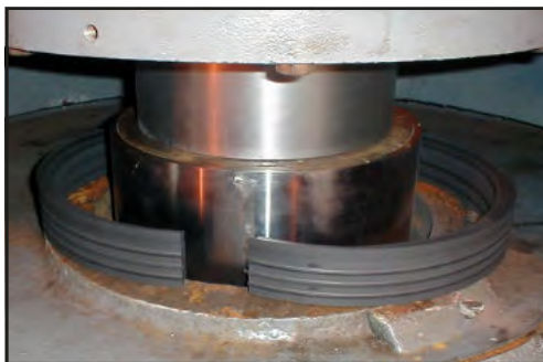
SpiralTrac installation in a large influent pump at a wastewater treatment plant
